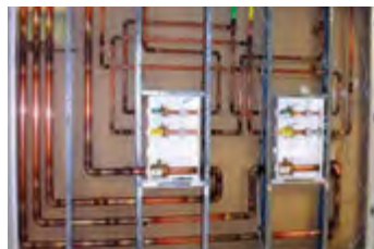
Medical Gas Pipeline
