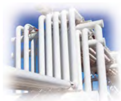
Industrial Gases Pipeline
